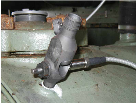
IPT-01XHT sensor installed on Kiene valve
